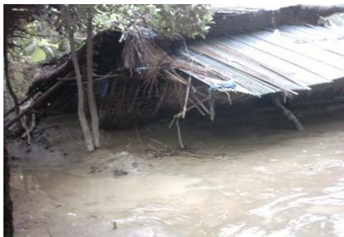
Existing House in the disaster prone area. (Damage during disaster)
